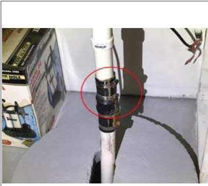
Sump pump check valve is leaking
