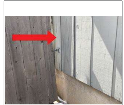
Rotten siding on south east corner
