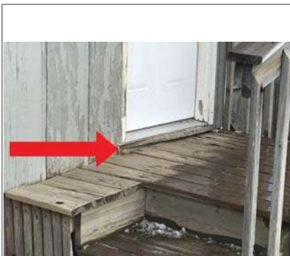
Threshold is rotten
