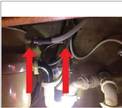
Corroded pipe, and dishwasher connected to disposal. Recommend separate drain or air gap.
