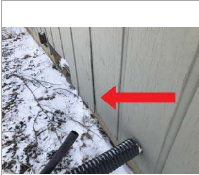
Recommend securing siding
